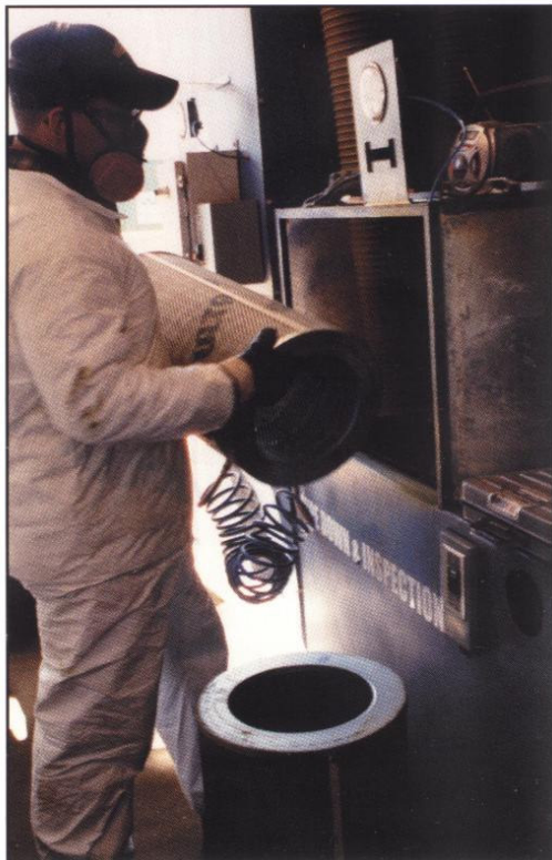
Good-as-new! The operator places a torit filter into the machine that vacuums the debris. The self-contained cleaning system spent a two-week period on-site to clean filters.
